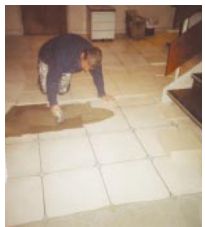
Ardurit S38 being trowelled to provide ribbed bed for the new tiles
